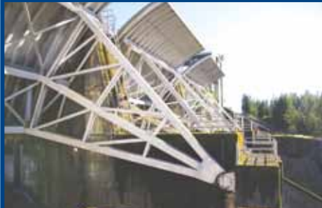
RADIAL SPILLWAY GATE TRUNNION BUSHINGS
