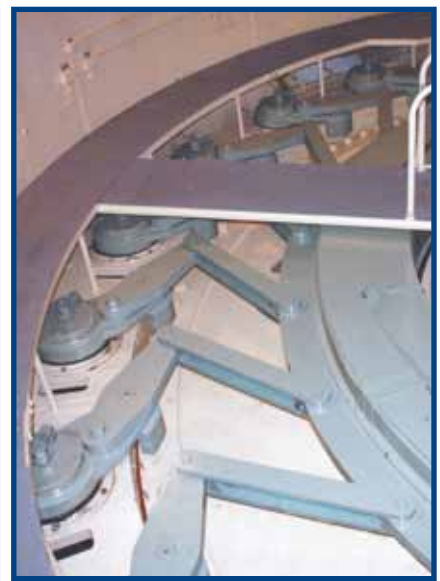
WICKET GATES WITH CIP HYDRO
